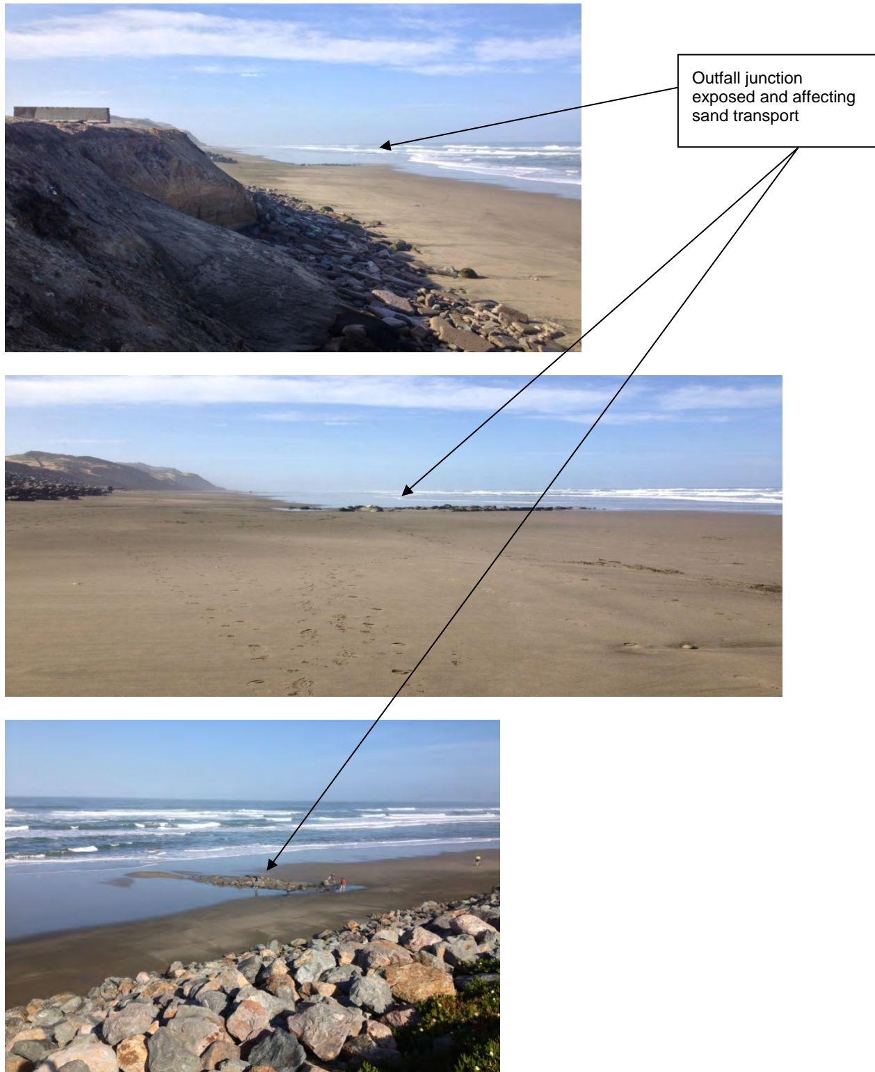
Figure 13: The sewer outfall pipe crosses SOB in front of the sewer plant. The top of the outfall junction structure has been visible in the winter since the late 1990s. It is located just south of the erosion hotspot where sand was placed in early 2000s, and just north of the location of the emergency revetment constructed in 2010. Photographs, April 30, 2013 Bob Battalio.
