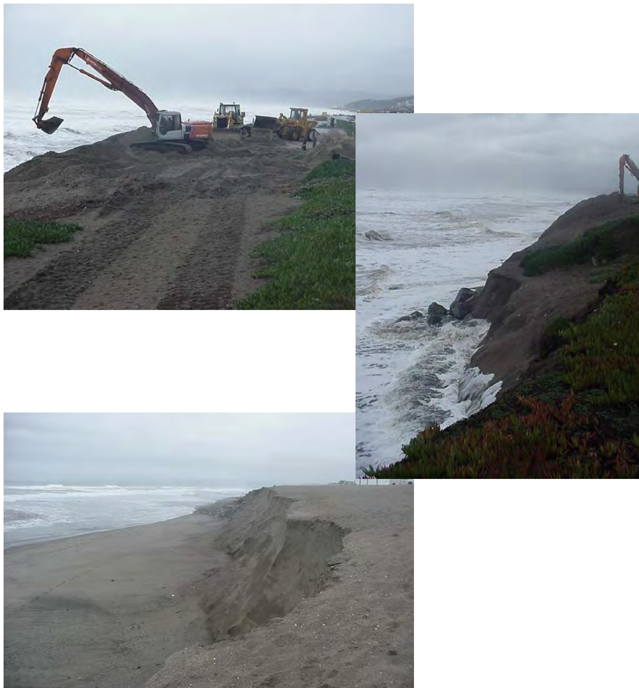
Figure 15: Sand placement in the form of a sacrificial sand berm at SOB in 1999-2000. The location is between the SWOO and the south Parking lot, with some sand placed south of the SWOO. The SWOO is under the quarry stone seen in the middle picture. The south parking lot is adjacent to the concrete rubble in the lower picture and behind the construction equipment in the upper picture. Photographs, Bob Battalio.
