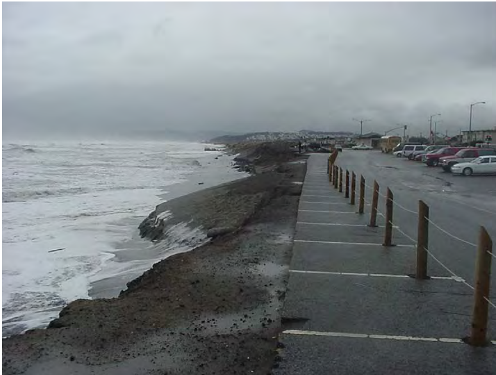
Figure 9: South Ocean Beach: Top: Post construction in 1990s. Bottom: eroded in early 2000s. The wood posts (top photo) were removed by erosion, and were replaced in the parking remaining parking lot (bottom photo). Photographs, Bob Battalio.
