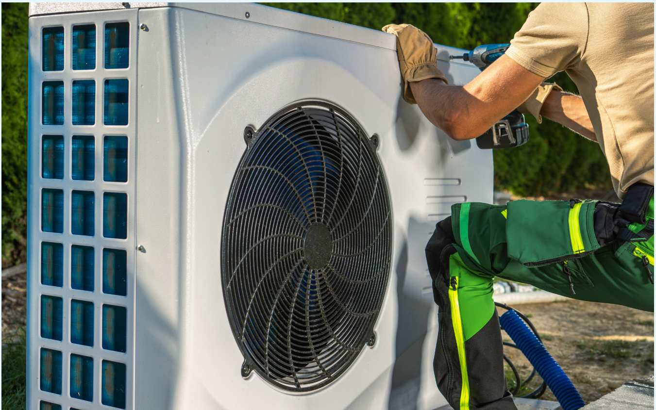
Heat pump installation
